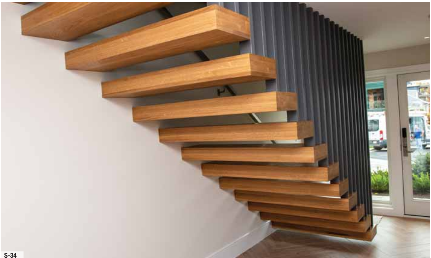
S-34 Stair structure is hidden in the wall and supported from the ceiling
